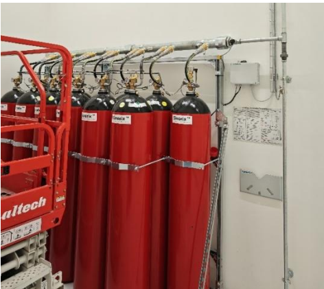
© safetyfocus GmbH – Fire-extinguishing battery
